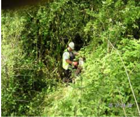
The winch was located over 200m away from the unit in a very remote area of woodland, no vehicle access at all. Our brave winch man managed to position the winch over the manhole without too much injury from the brambles and nettles
