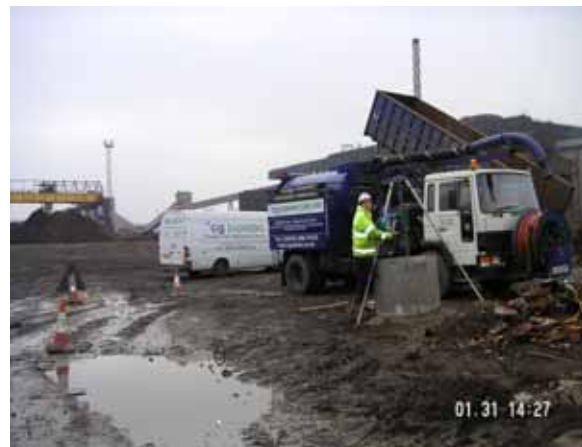
Area cleared of scrap with a new manhole ring to prevent metal being pushed back into the manhole, the heap of debris at the side of the manhole was the type of material taken out.
